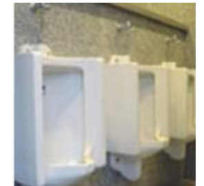
Urinals and urinal flush valves
